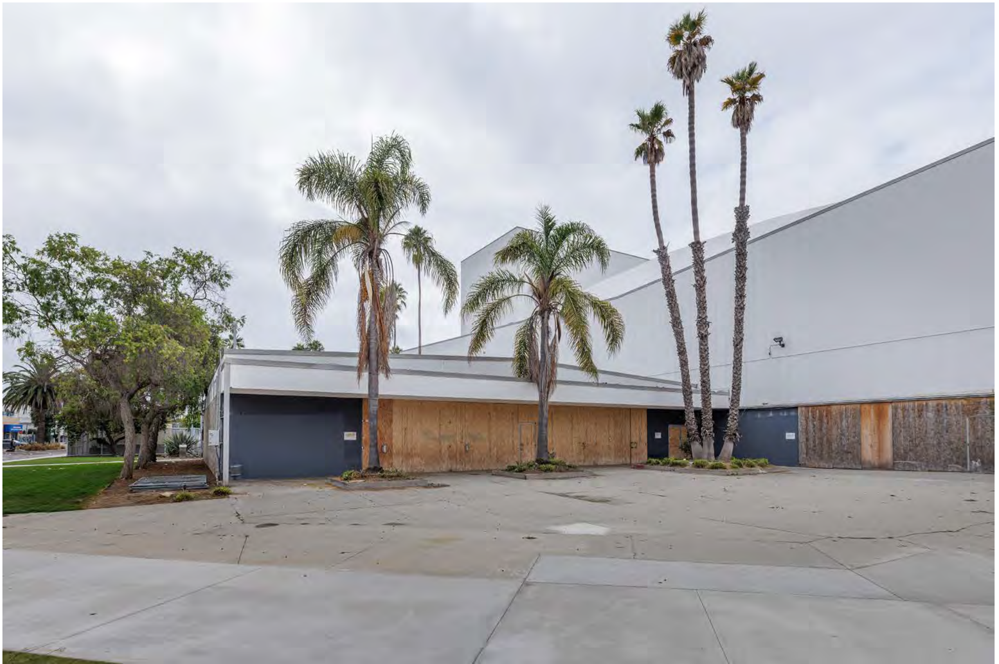
CA_LOS ANGELES COUNTY_SANTA MONICA CIVIC AUDITORIUM_0004.TIF EAST WING NORTHWEST ELEVATION, CAMERA FACING SOUTH.
