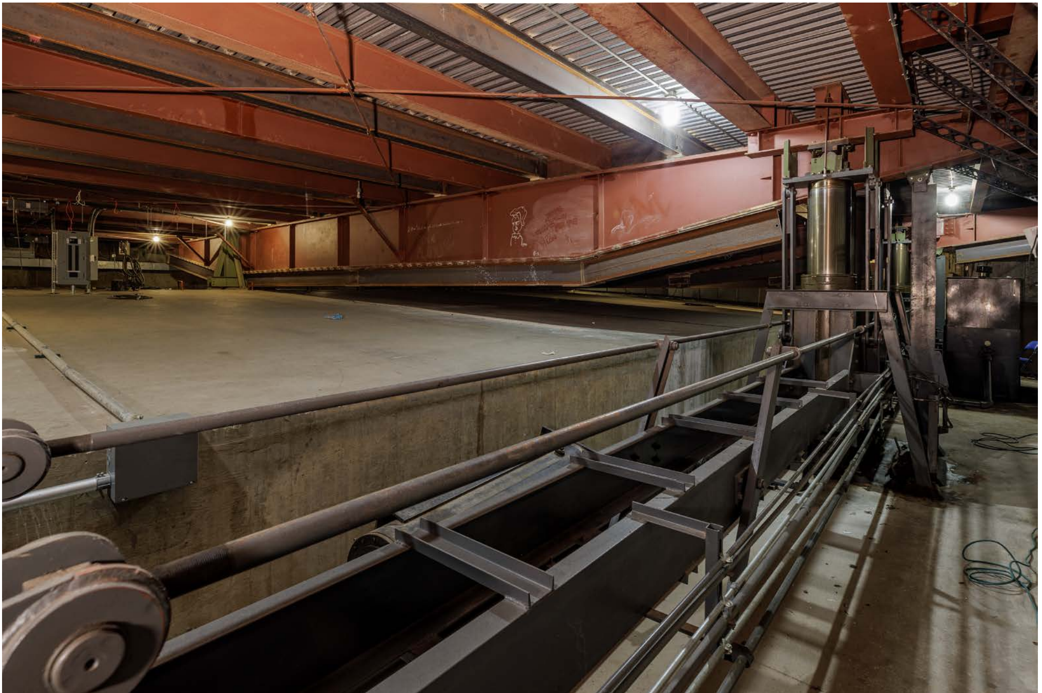
CA_LOS ANGELES COUNTY_SANTA MONICA CIVIC AUDITORIUM_0022.TIF INTERIOR BASEMENT: TILTING FLOOR (ABOVE), HYDRAULIC PISTONS (RIGHT), CAMERA FACING NORTH.
