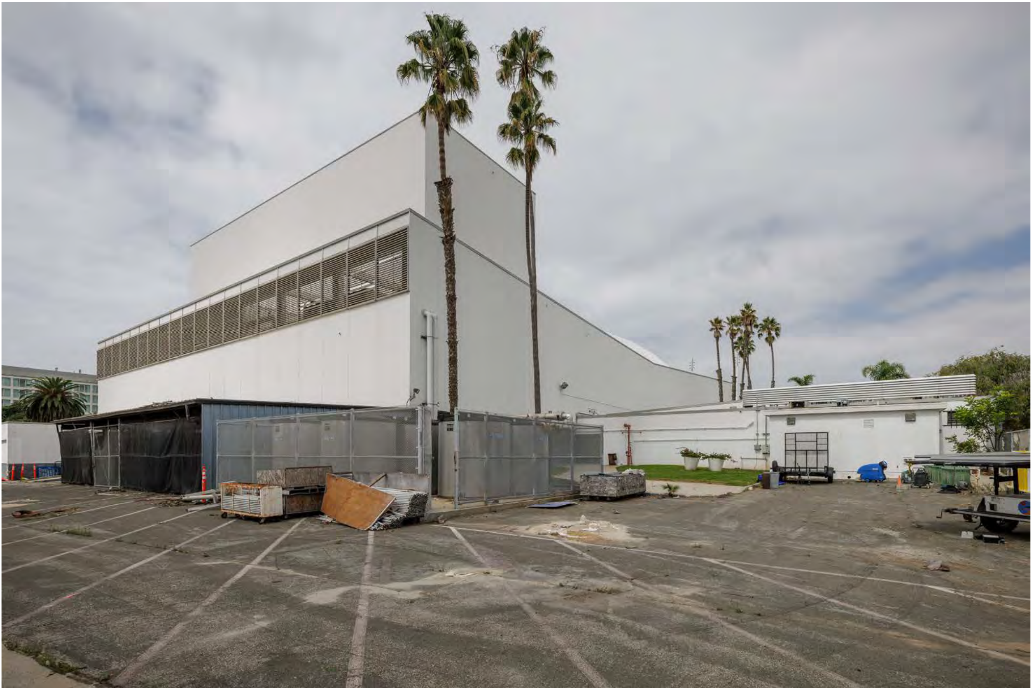
CA_Los Angeles County_Santa Monica Civic Auditorium_0005.tif SOUTHEAST/REAR ELEVATION (LEFT), REAR OF EAST WING (RIGHT), CAMERA FACING WEST.
