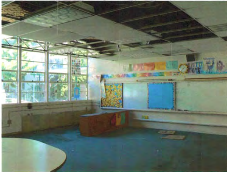
Plate 113. Classroom Interior (Fire Damaged)
