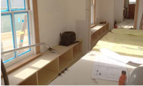
Bookcases under the south windows will have cushions to provide extra seating.
