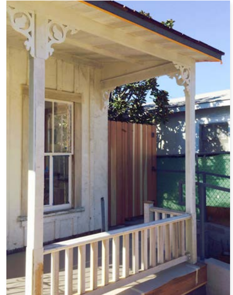
Reconstruction of the railings and the corbels make a big difference in the rehabilitation of the porch. Photo by Carol Lemlein
