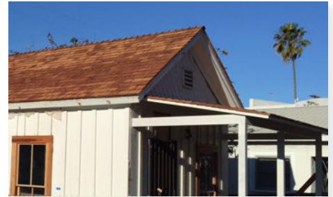
The reconstructed porch, new shingled roof and windows are visible above the construction fence.
