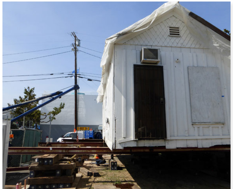
The house was supported on a set of steel beams and railroad ties to give the workers room to build the foundation under the house.
