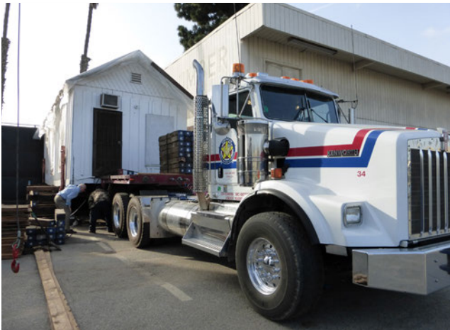
Getting the Shotgun House ready to move took several hours of preparation. The house was lifted and supported with railroad ties so the flatbed trailer could be rolled beneath it.
