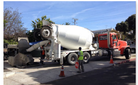
May 1, the cement truck rolled in and the crew poured the first sections of the foundation. Once the concrete set, the wood forms were removed, and they moved on to the porch foundation.
