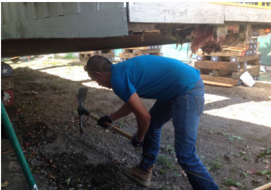
The trenches for the foundation were dug by hand. Trenches were also dug for the foundation of the porch and the addition that will be built on the back of the house.
