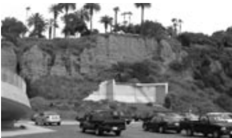
Foundation still embedded in the cliff at the 800 block of PCH, photo by Dick Orton
